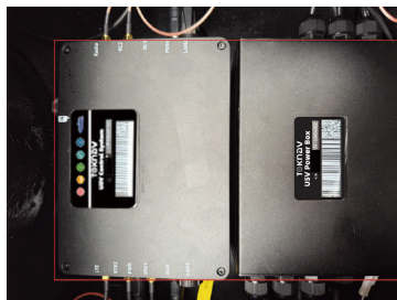
Figure 1.3.2 the Control System and USV Power Box of Tboat20
