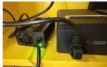
Figure 14.7 Battery Fully Charged Status
